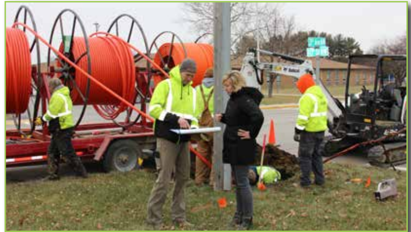
Erich Gamm, the owner of West Union Trenching, describes the fiber boring and connection process to Hollee McCormick during a visit to Allamakee County in December 2020.
